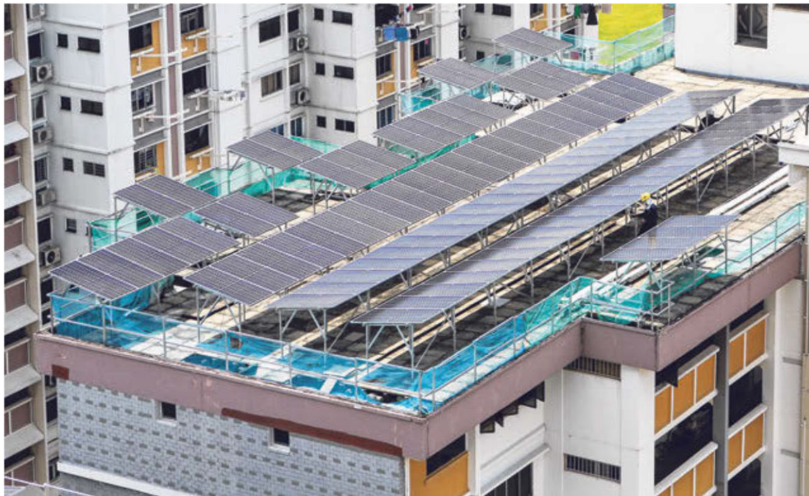
Solar panels on HDB rooftops. Singapore can increase efforts to develop and test-bed sustainable innovations – from green energy to waste management to carbon capture – that can later be diffused throughout the region. BT FILE PHOTO
