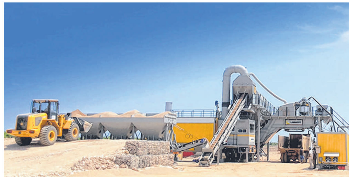
The Linnhoff MobileMix Asphalt Mixing Plant TSD1500 is a popular choice in the Trans-Sumatra Toll Road Project in Indonesia due to its ease of mobilisation and demobilisation. PHOTO: LINTEC & LINNHOF ASPHALT
