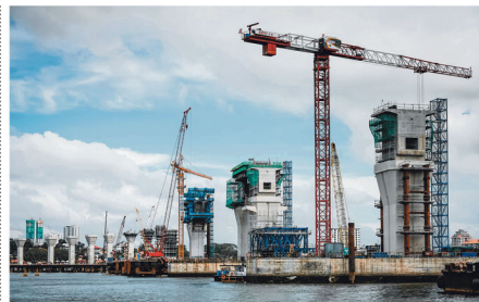
Work on the Johor Bahru-Singapore Rapid Transit System Link marine piers is well under way. ST PHOTO: GAVIN FOO
