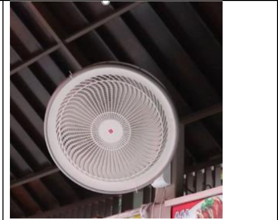
Wall-mounted fan powered by the AD system
