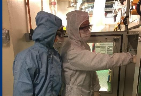
Mr Gabriel Chen and Mr Leong Chee Meng performing inspection on a gas detection system on 31 Oct 2018.
